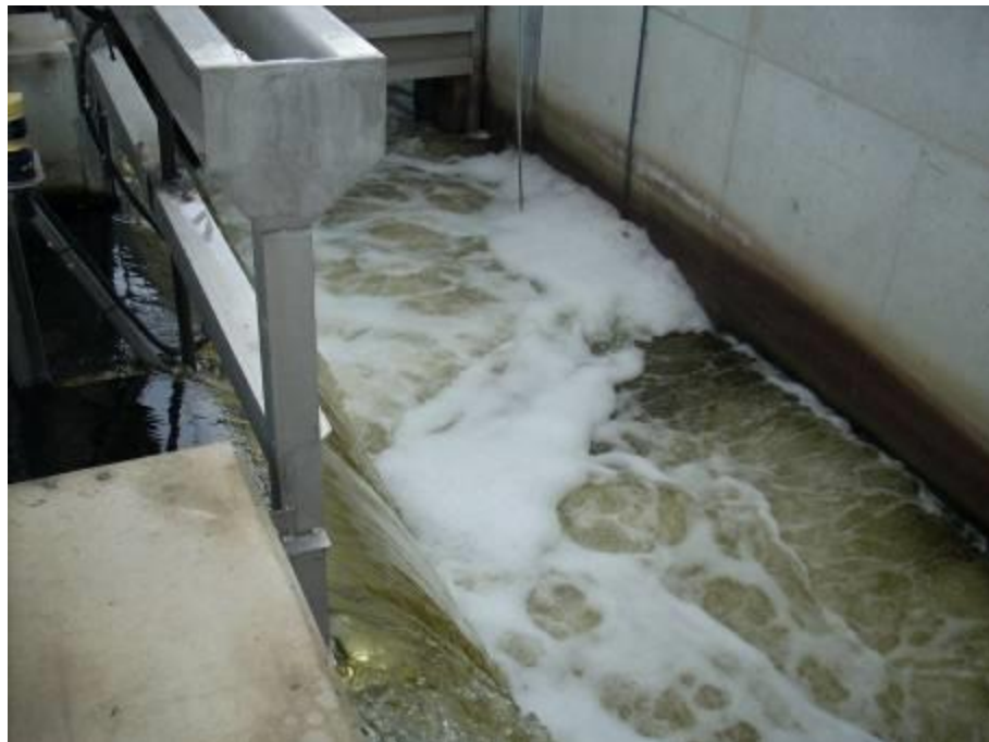
Figure 14 Oxley Creek WWTP post UV.
