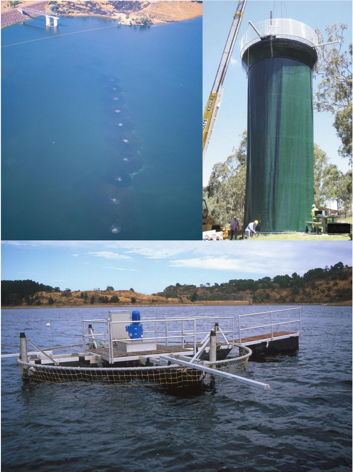
Figure 1. Destratification systems. Clockwise from top left: 10 bubble plumes at Chaffey Dam, NSW; WEARS draft-tube mixer awaiting deployment (photo courtesy WEARS); WEARS mixer deployed at Myponga Reservoir, SA.
