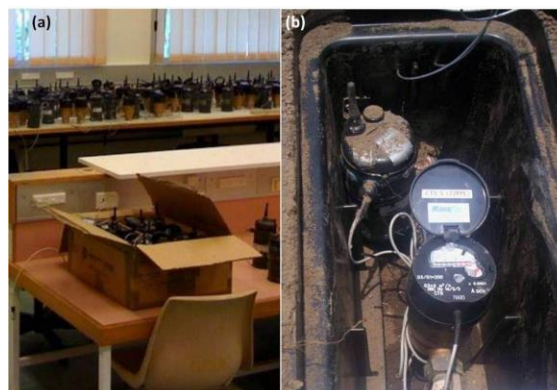
(a) Each meter/data set was individually configured. (b) Installed smart meter and data logger.
