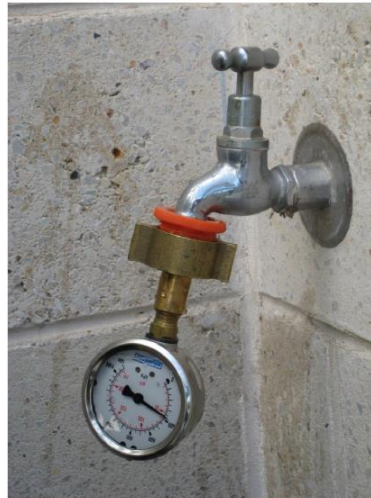
Figure 8: Pressure measurement at an external tap to confirm water flow from a rainwater tank.
