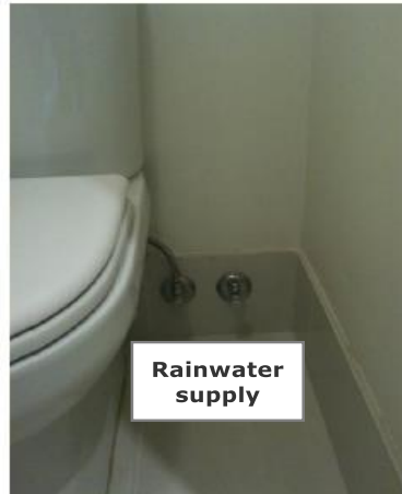
Figure 6: An example of a rainwater supply connection that fills the toilet cistern.
