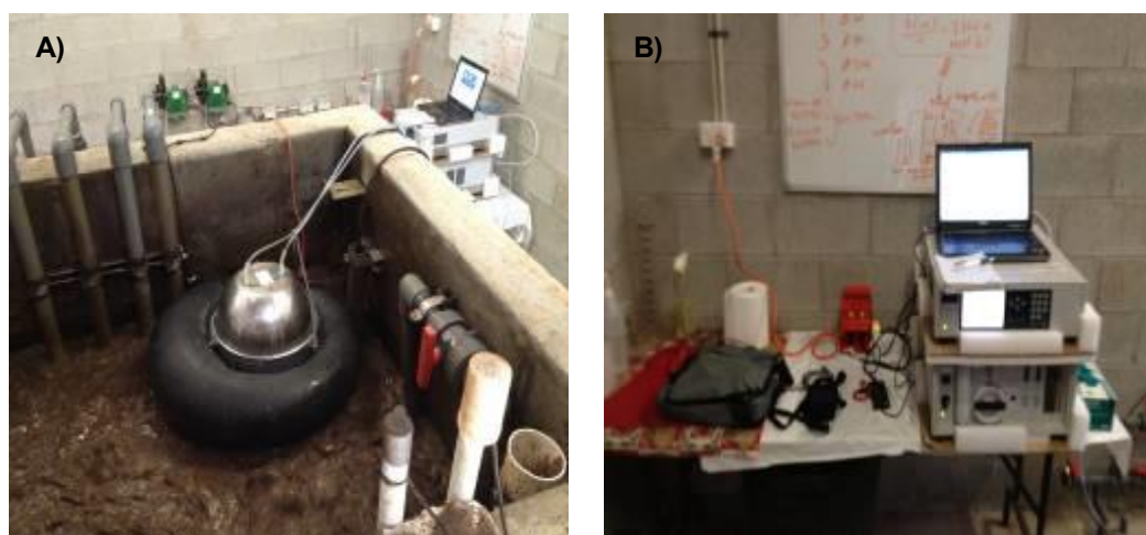
Figure 29: Example deployment of the gas analysis system in the field – A) The flux hood on top of the CDM MBR aeration tank; B) The gas analysis and data collection workstation.
