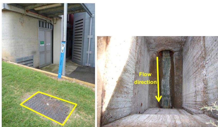
Figure 9. External and internal view of the selected manhole (0.8mx0.4mx1.0-1.3m) in front of Ipswich Hospital.
