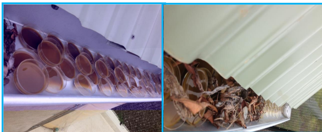
Figure 8. Possum faecal slurry in the gutter.
