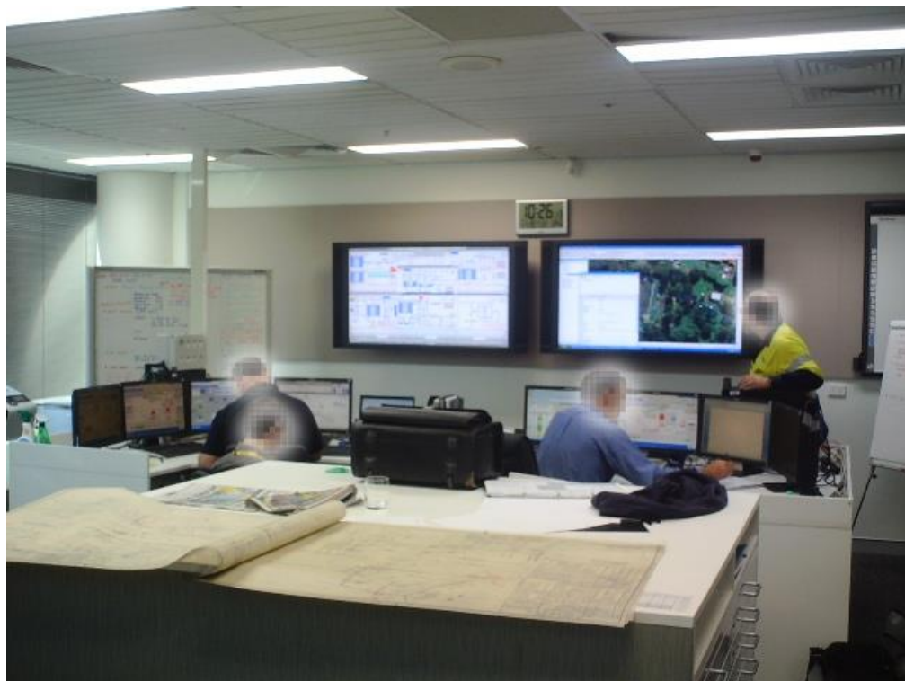
Figure 1: The control room at the BWTA central office, showing two operator consoles with four monitors each, and two large wall-mounted LED screens.
