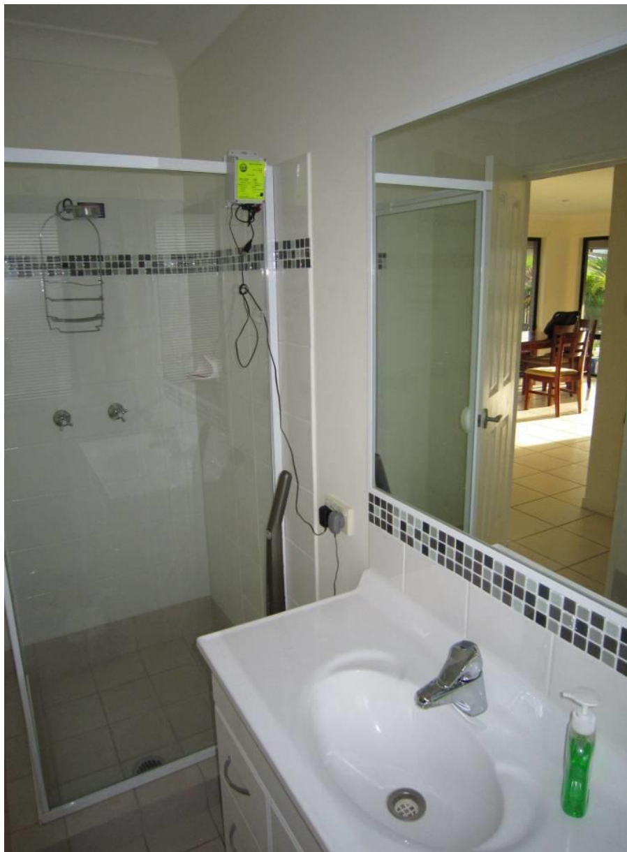
Figure 4: Acoustic sensor in ensuite.
