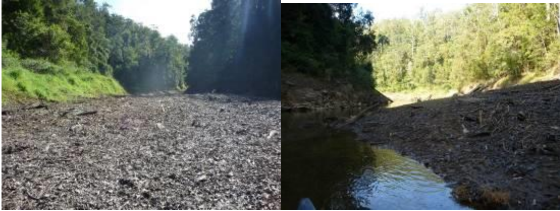
Figure 26: Accumulation of coarse woody debris at upstream end of Little Nerang Dam. Photos courtesy A. Grinham.
