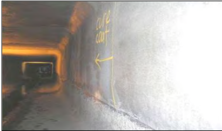
Figure 2. CAC Application Trial in SWSOOS 2007, SW showing minor crazing after 18-19 years of service, otherwise intact and in good conditions.
