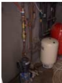
pump and associated equipment in basement plantroom
