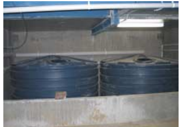
tanks located at end of basement
