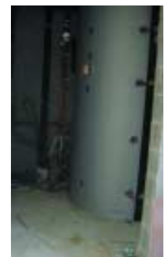
solar boiler and associated equipment in basement plantroom
