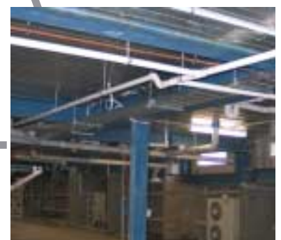
rainwater supply pipework attached to underside of ground suspended slab
