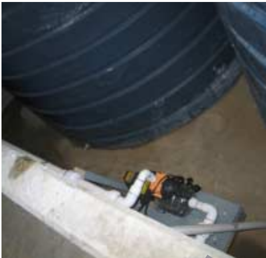
pump and associated equipment in basement
