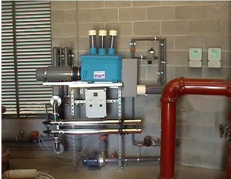
Figure 5 System control and filter equipment
