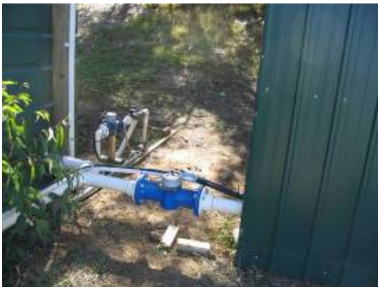
Water meters at the balancing stores
