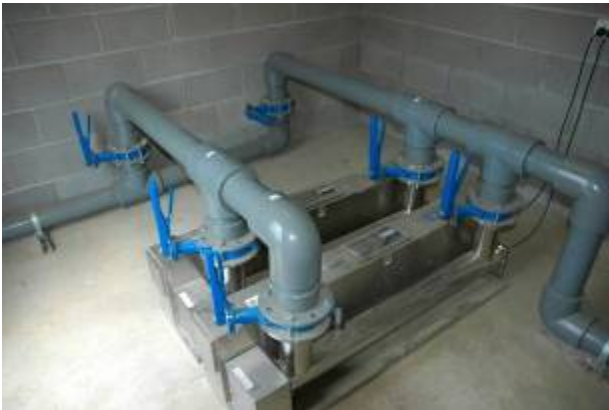
UV disinfection units
