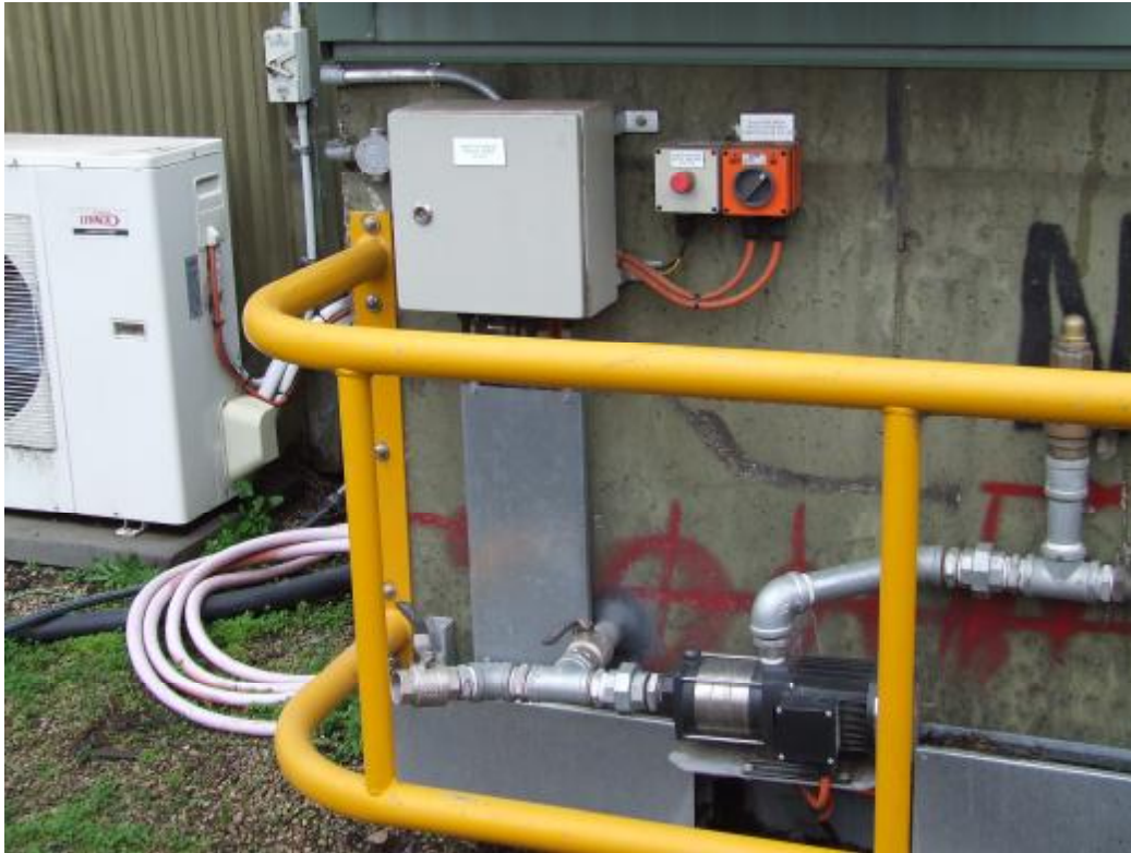
Recirculating pump and associated controls mounted at discharge end of settling tanks.
