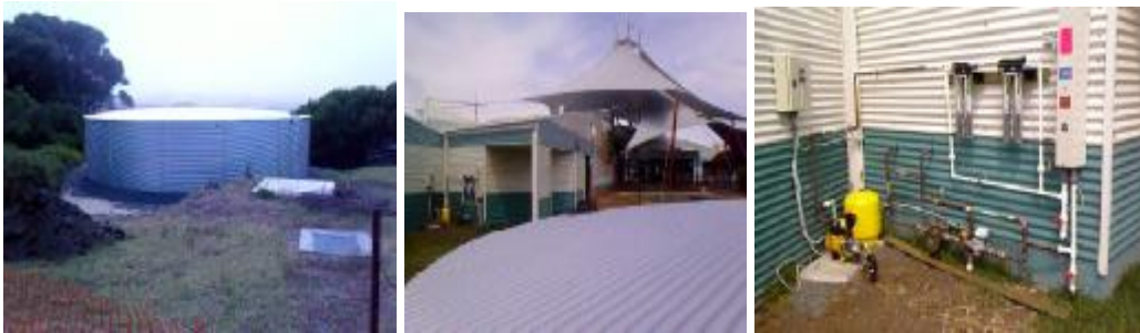
Main Water Tank at Penguin Parade Proximity to Visitor Centre Pumps and mains back up materials
