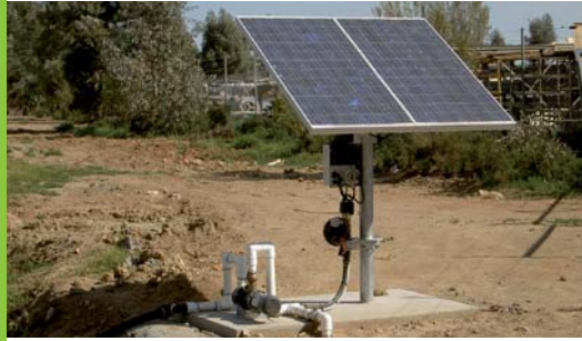
Solar pump and panel
