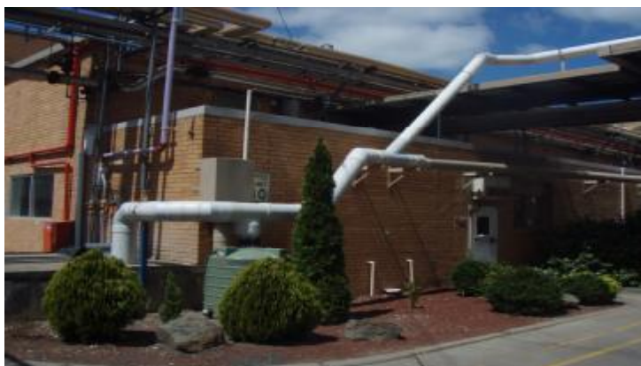
Pipework, first flush tank and pumping station Noodle and Pizza roof
