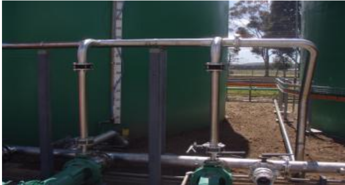
Backflow prevention device
