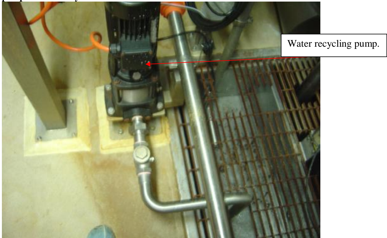
Figure 7.2.5: Water recycling pump. Returning seal water to xxx.
