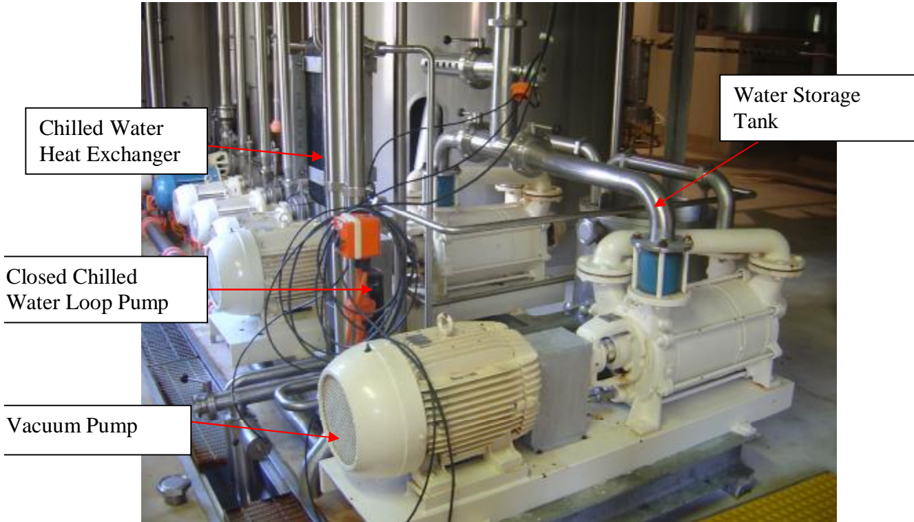
Figure 7.2.1: Closed chilled water loop on CD2 vacuum pumps.
