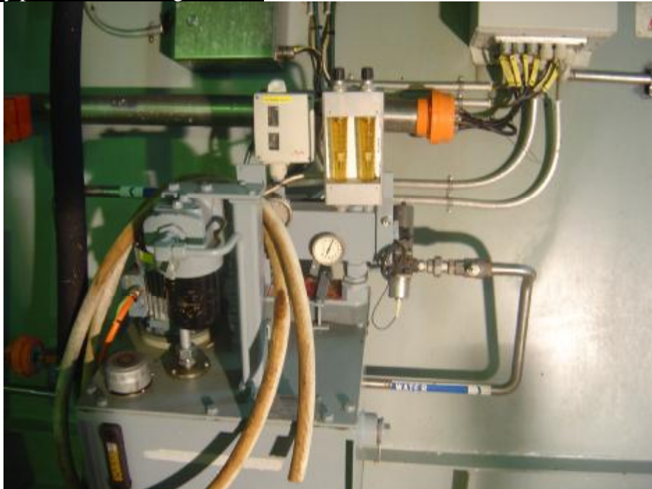
Figure 7.1.5: MSD2 MVR fan, oil cooling system, showing the inlet and outlet of water from the plate heat exchanger. Note the MSD2 MVR cooling water is recovered to the water recovery pit shown in figure 7.1.4, the CD2 MVR's cooling water has been placed on a closed chilled water loop.
