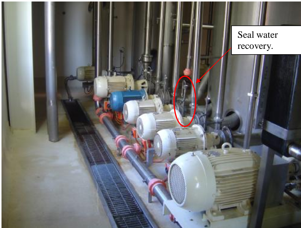
Figure 7.2.2: Seal water recovery on evaporator pumps.
