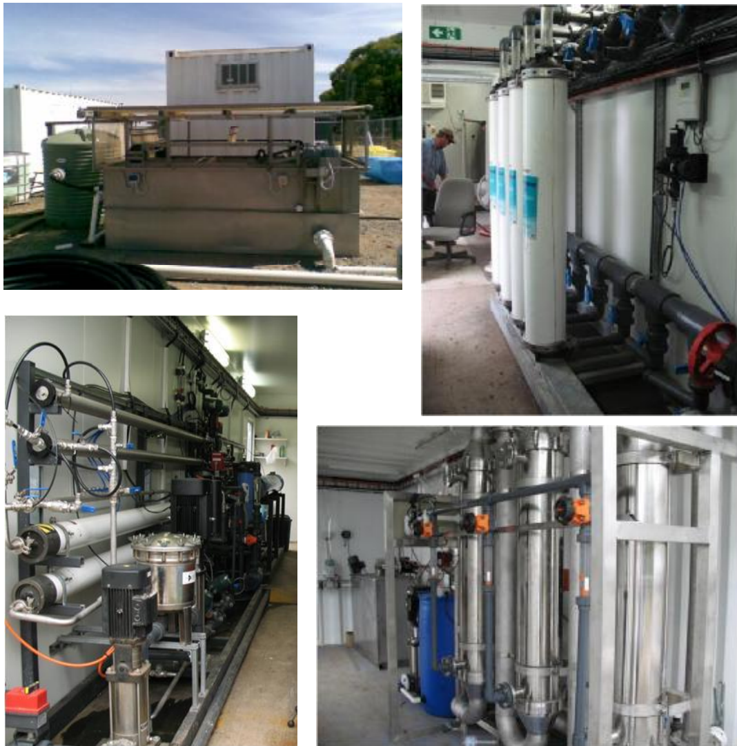
Figure 2.1.2: Pilot Plant component, DAF (top left), UF (top right), RO (bottom left) and ASP-CUF (bottom right).
