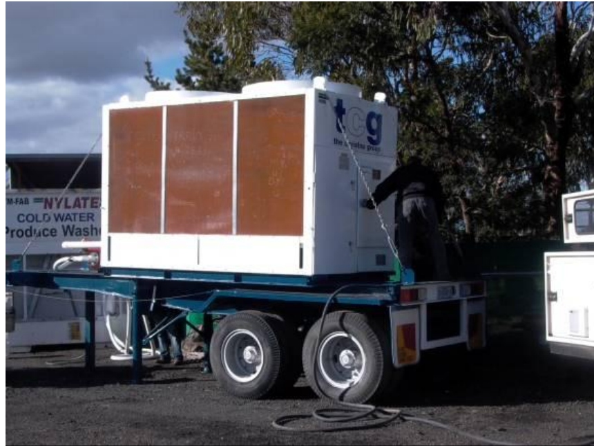
Figure 3.4. The water chilling unit associated with the Smart Water hydrocooler.
