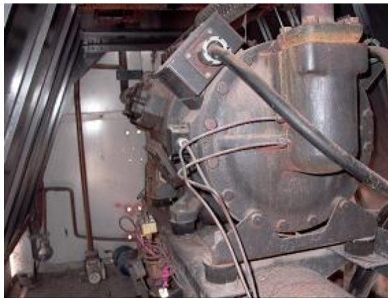
Figure 5.3. The compressor used in the water chilling unit.
