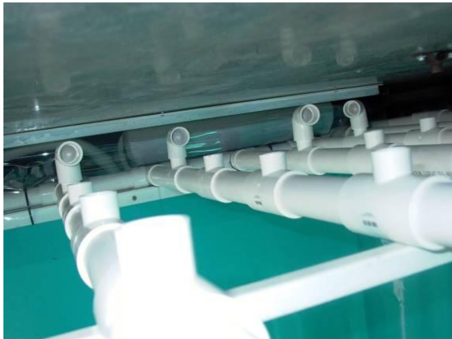
Figure 3.5. A view of the water distribution system in the roof of the shipping container. Water puthers out of the upwards-facing tee-pieces. The inwards facing bends at the rear of the photograph help to ensure that the water is directed towards the produce.
