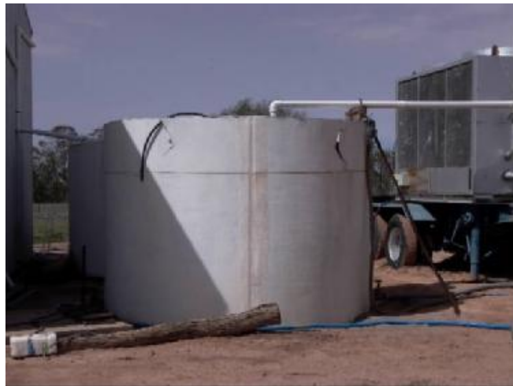
Figure 5.5. The tank used to store chilled water when the cooling unit was located at a property in Goondiwindi, Queensland. The pipe leading from the chilling unit can be seen replenishing the tank. The blue hose on the ground leads to the hydrocooler.
