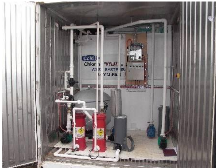
Figure 3.11. The general layout of the filter room showing the blue Ebara DW 400 pump that is used to pump water from bay 1 to one of the water distribution arrays. The green Onga pump draws water from bay 1 whence it is strained and distributes it to tank 2 thus promoting mixing. The photograph shows the stainless steel strainer in the filtration and chemical dosing system removed from its housing. Water leaving this strainer is pumped by an Onga pump to the sand filter – the grey, almost spherical component on the left of the figure. The cylinders that contain the disinfectant, bromo-chloro-dimethylhydantoin, are red.
