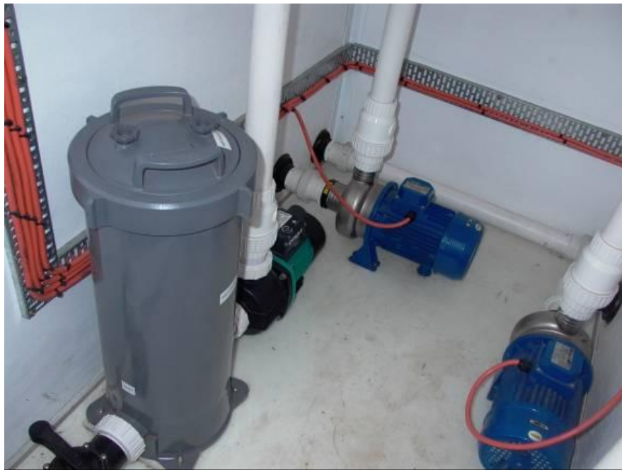
Figure 3.13. The pump room located between bays 2 and 3. Water from bay 2 is strained before being pumped by the green Onga pump to tanks 5 and 6. The blue Ebara pump near the centre of the figure pumps water from the reservoir of Bay 2 to the water distribution system that is located above Bay 2.
