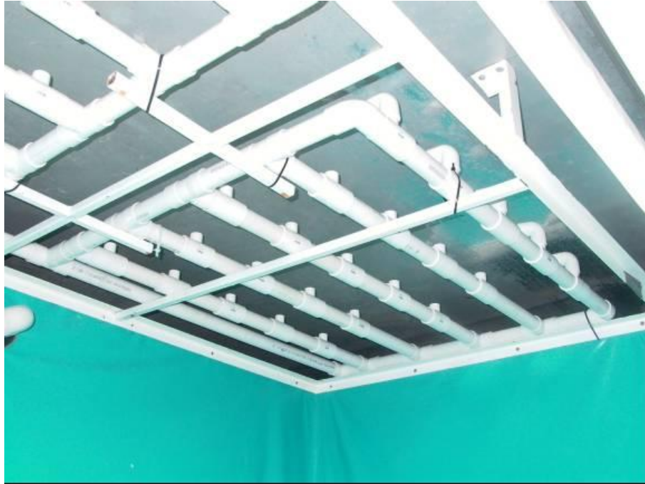
Figure 3.6. A view of the water distribution system from below. It is supported by a light metal frame.
