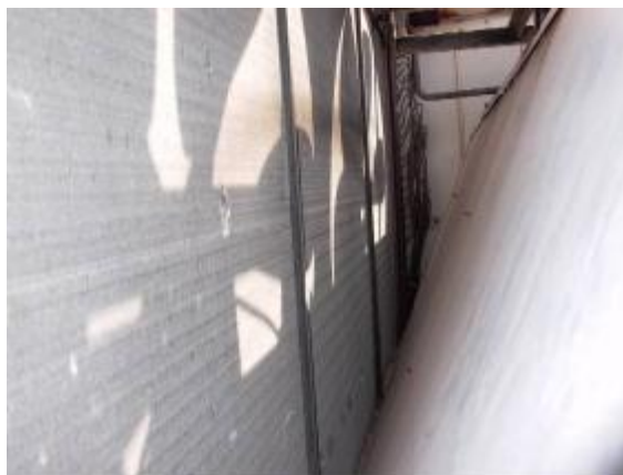
Figure 5.4 The finned coils on the left hand side of the photograph constitute the condenser of the water chilling unit.
