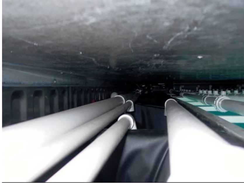
Figure 3.14. Pipes carrying chemically dosed, filtered and water from Bay 1 to the water tanks located at the rear of the hydrocooler. The pipes are laid over the water tanks located at the rear of the hydrocooler.
